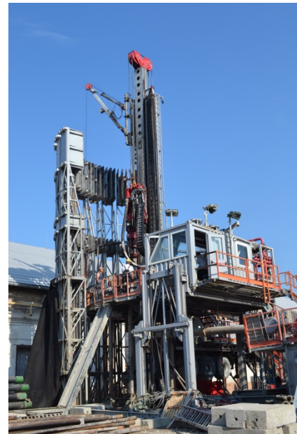
Directional well drilling in Szeged, one of the CROWD THERMAL case studies. Credit: SZETAV Ltd.
